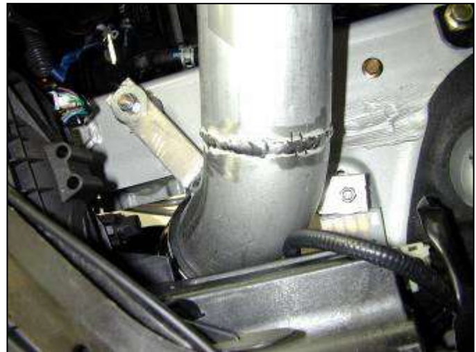
i. Secure the pipe with the supplied washers and lock nuts. Do not completely tighten lock nuts.
